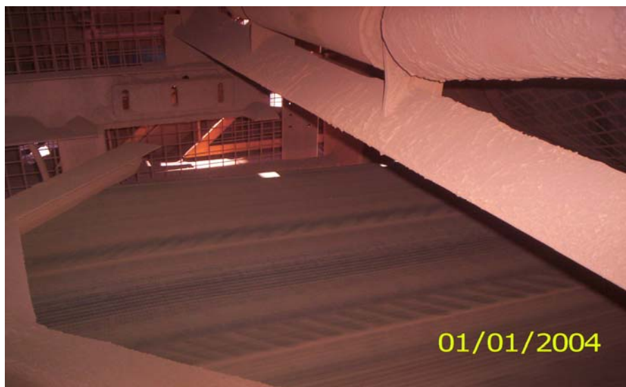
The above belt has exposed cables in the centre of the bottom cover, top cover fine
