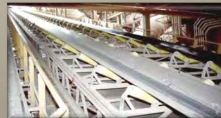
900 TPH Raw Meal Handling Conveyor System
