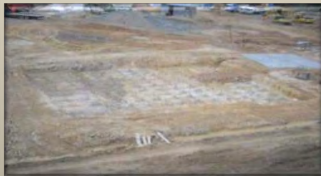
WATER PUMP HOUSE PEDESTALS
