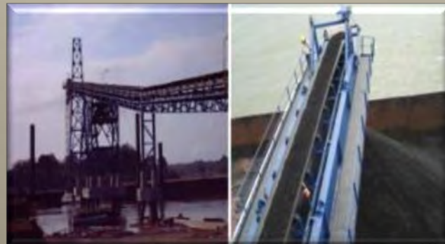
TEPIAN ULAK / PIK BARGE LOADING SYSTEM
