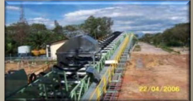
DUMAI FIBRE, SHIP LOADING SYSTEM
