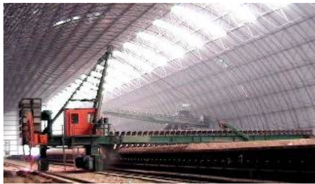
Stacker in shed
