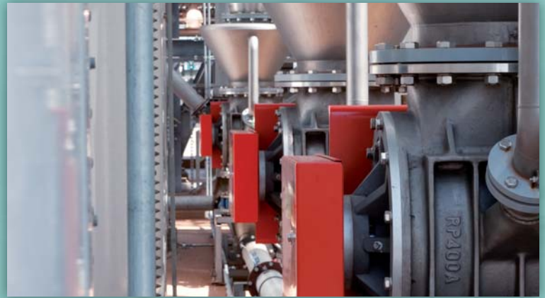
Rotary Valve Stations
