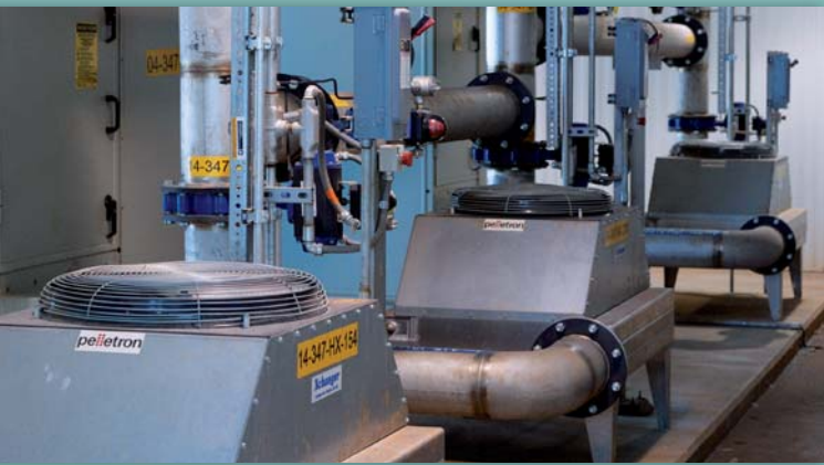
Blower Stations And Heat Exchanger
