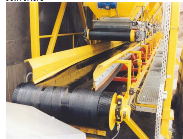
Concrete Mixer Plant - drives controlled by frequency converters
