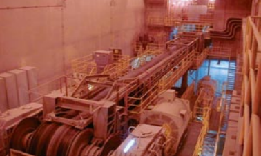
Drive station at downhill ore conveyor system
