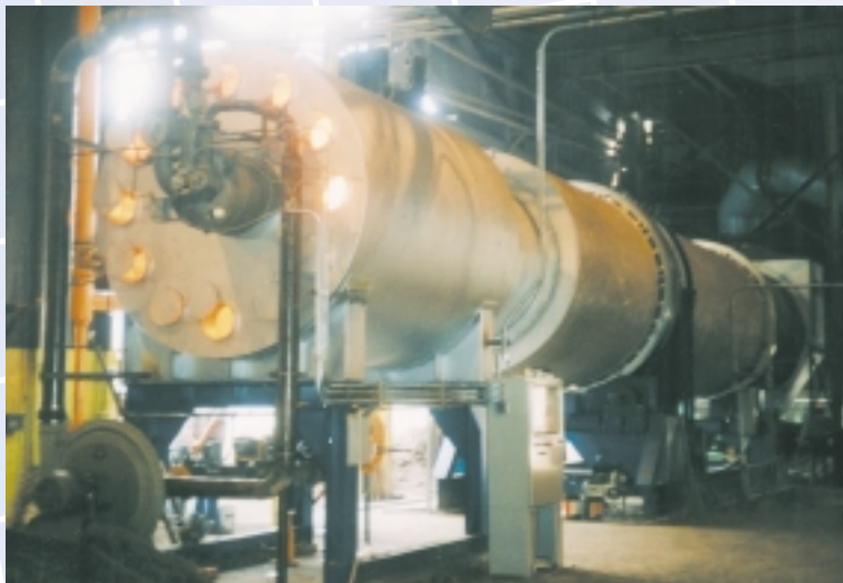
A Rotary Dryer and Combustion Chamber
