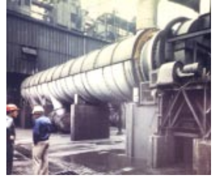
Indirect rotary dryer for processing carbon black
