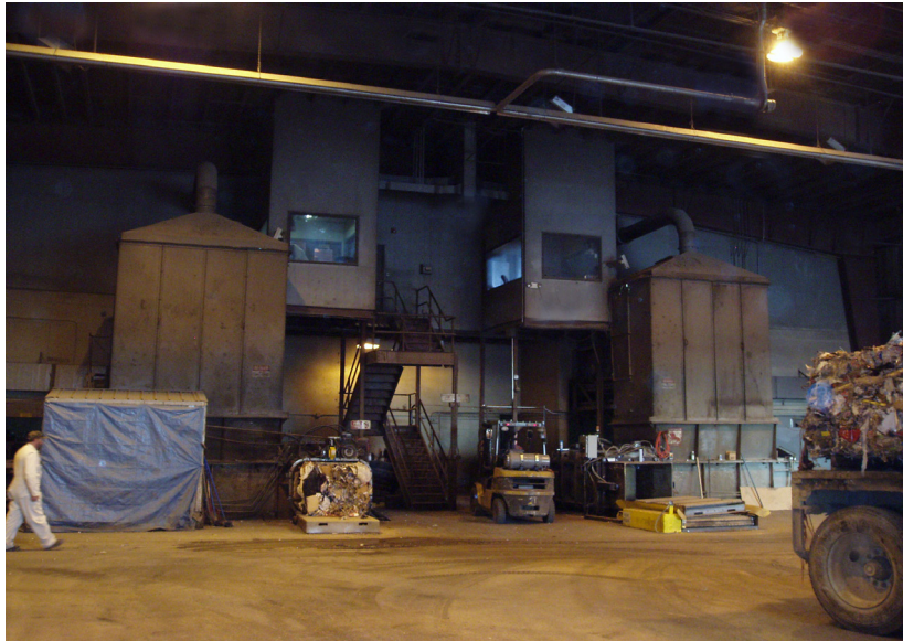
Overview of the two Balers
