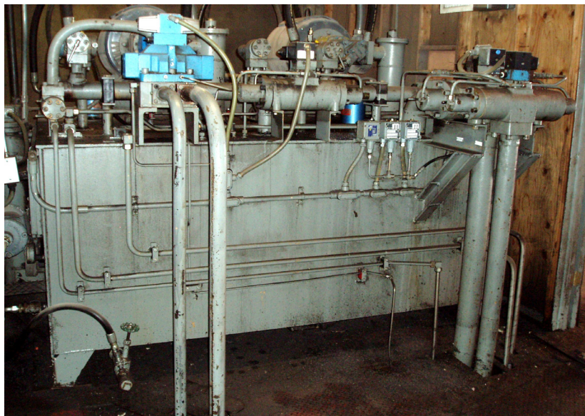
Hydraulic Power Unit (Two - 100 Hp Motors)
