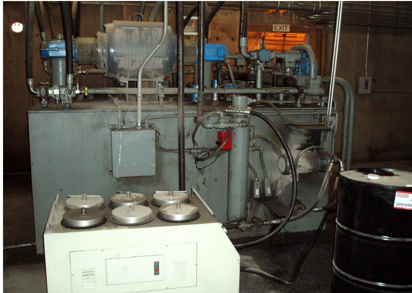
Hydraulic Power Unit (Two - 100 Hp Motors)
