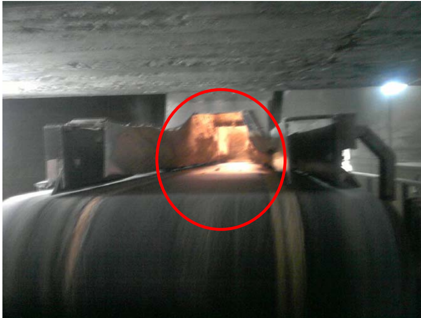
Front View of the Belt Conveyor
