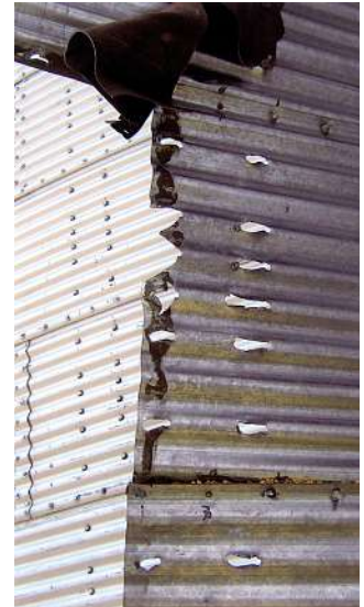
Fig. 5: Line of rupture to left of Fig. 3.
