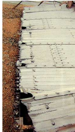
Fig. 4: Line of rupture of wall to right of Fig. 2.
