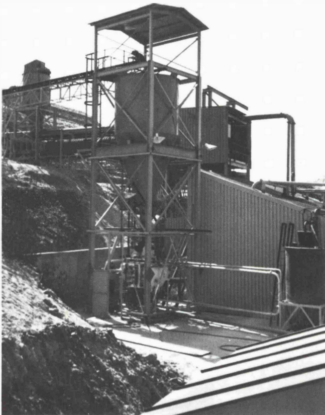
Fig. 7: View of feeding system for pneumatic conveying of dried gold slimes over 2,000 m for backfilling of gold mines
