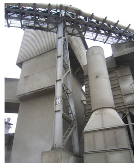
Beumer perfectly integrated the pipe conveyor into the existing system.
