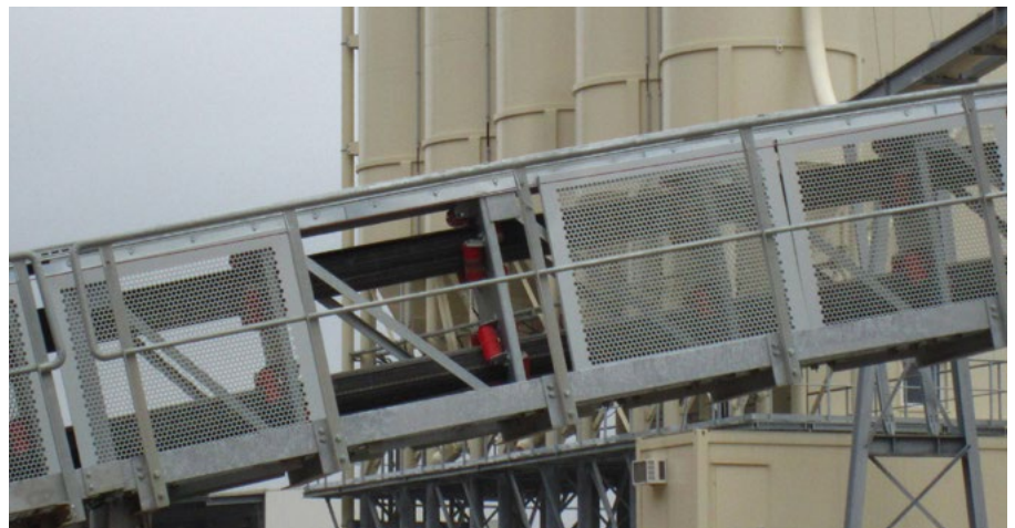
For accident prevention and safety requirements, the walkway side of the conveyor structure is covered with perforated plates.
