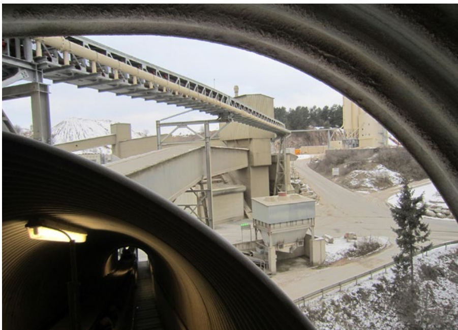
The connection of the pipe conveyor to the existing discharging point was a very challenging task.
