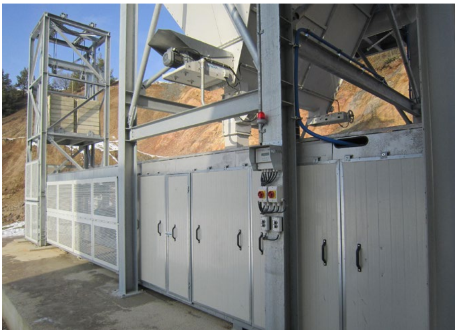
The take-up device is installed in the feeding area, where the customer is installing a dedusting unit.
