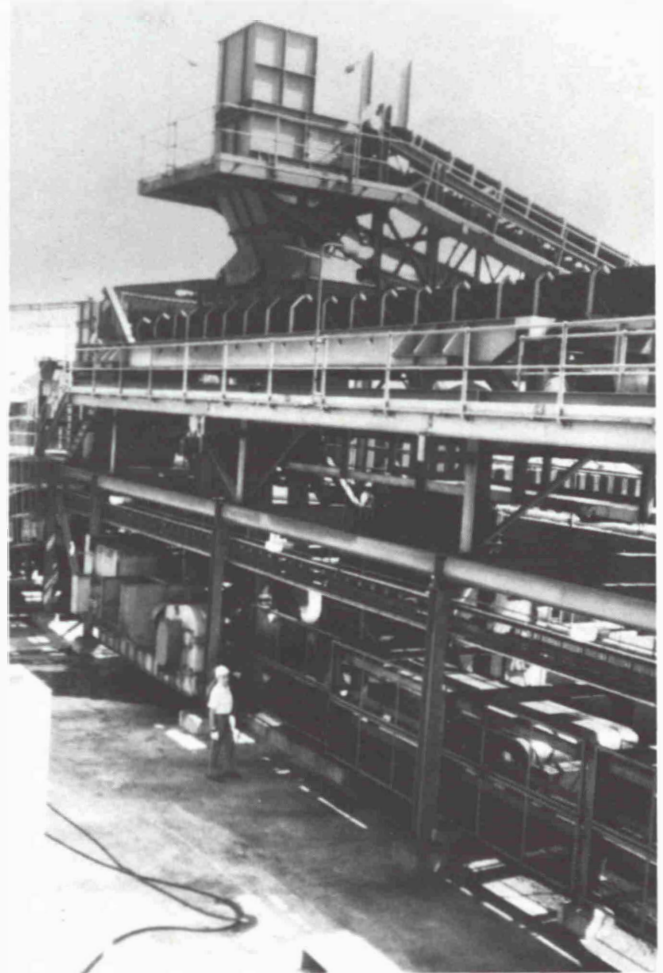
Fig. 12: Head end of recirculating conveyor and reversible yard conveyor drive station with moving head to permit future expansion.
