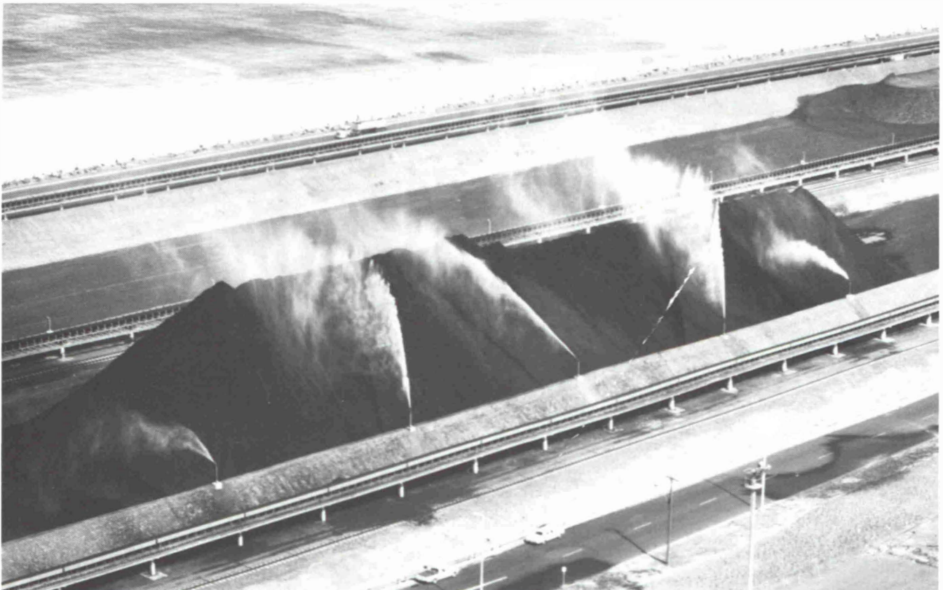
Fig. 7: All coal is treated with a chemical that binds free dust and forms a surface crust. Pioneering dual spray system is computer controlled on the basis of inventory, temperature, humidity, wind speed and direction. Yard conveyors are elevated for ease of clean-up.
