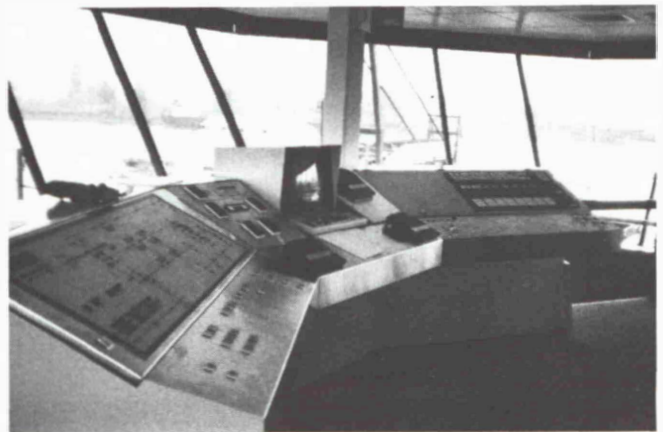
Fig. 13: Shiploading control tower with mimic panel, communication system and computer for programmable controllers, stockpile management, simulation, and data logging.
