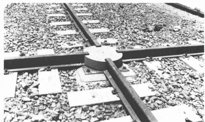
Fig. 23: Four jacking points are located at the cross travel tracks where the travel bogies are turned
