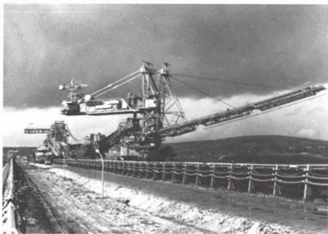
Fig. 16: PHB Weserhütte is building a similar crawler mounted luffing and slewing stacker as part of the final design of the system
