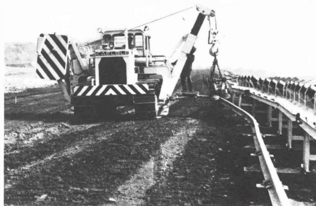
Fig. 15: Typical shiftable conveyor being shifted
