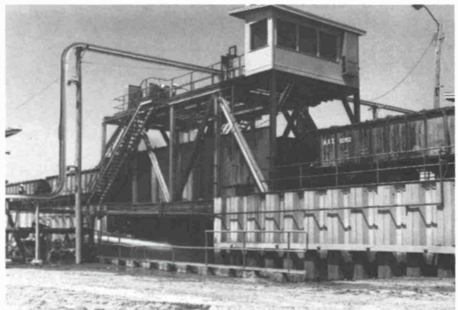
Fig. 7: Matrix from short-lived reserves is delivered to the Payne Creek washer in converted hopper cars. They are unloaded at a special matrix unloading hopper designed by Agrico. The car doors are opened over the hopper, and the matrix is blasted out of the cars with two remote controlled, moveable "hydraulicking" guns. The material hits a grizzly below the car, where it is slurried with a third gun, picked up by a pit pump, and piped to the nearby washer
