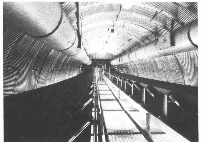
Fig. 1: Fling-designed shiploader allows efficient and economical loading of ocean-going vessels
