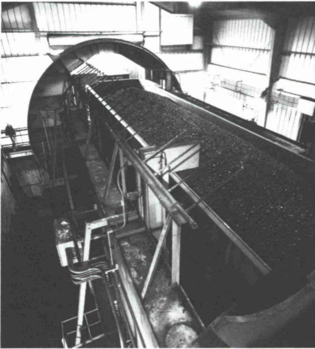
Fig. 12: Dust suppression system at car dumper installation
