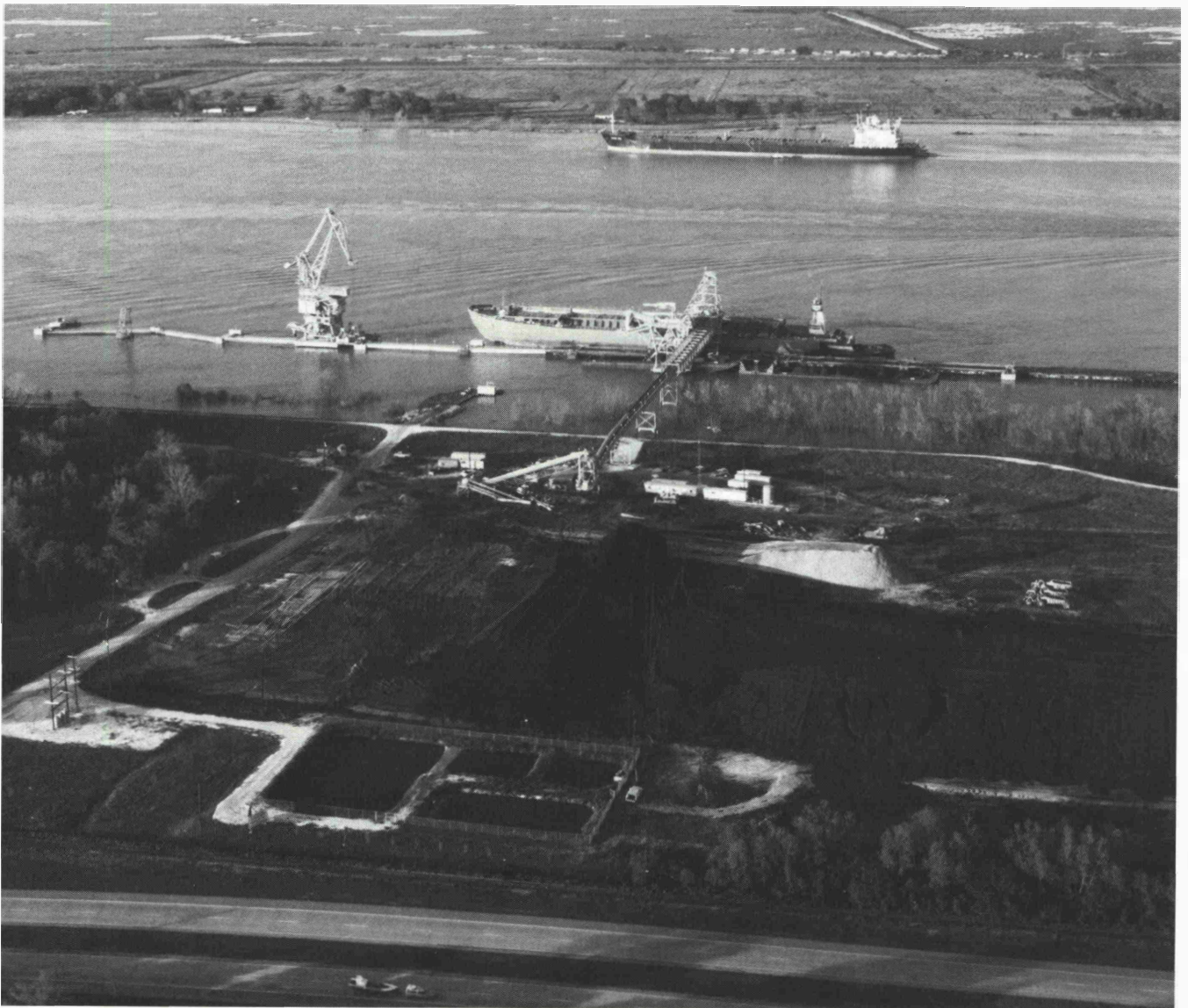
Fig. 13: Dravo designed these collection ditches surrounding the coal storage area and the retention pond to provide adequate drainage and treatment of stormwater runoff at Cora Dock
