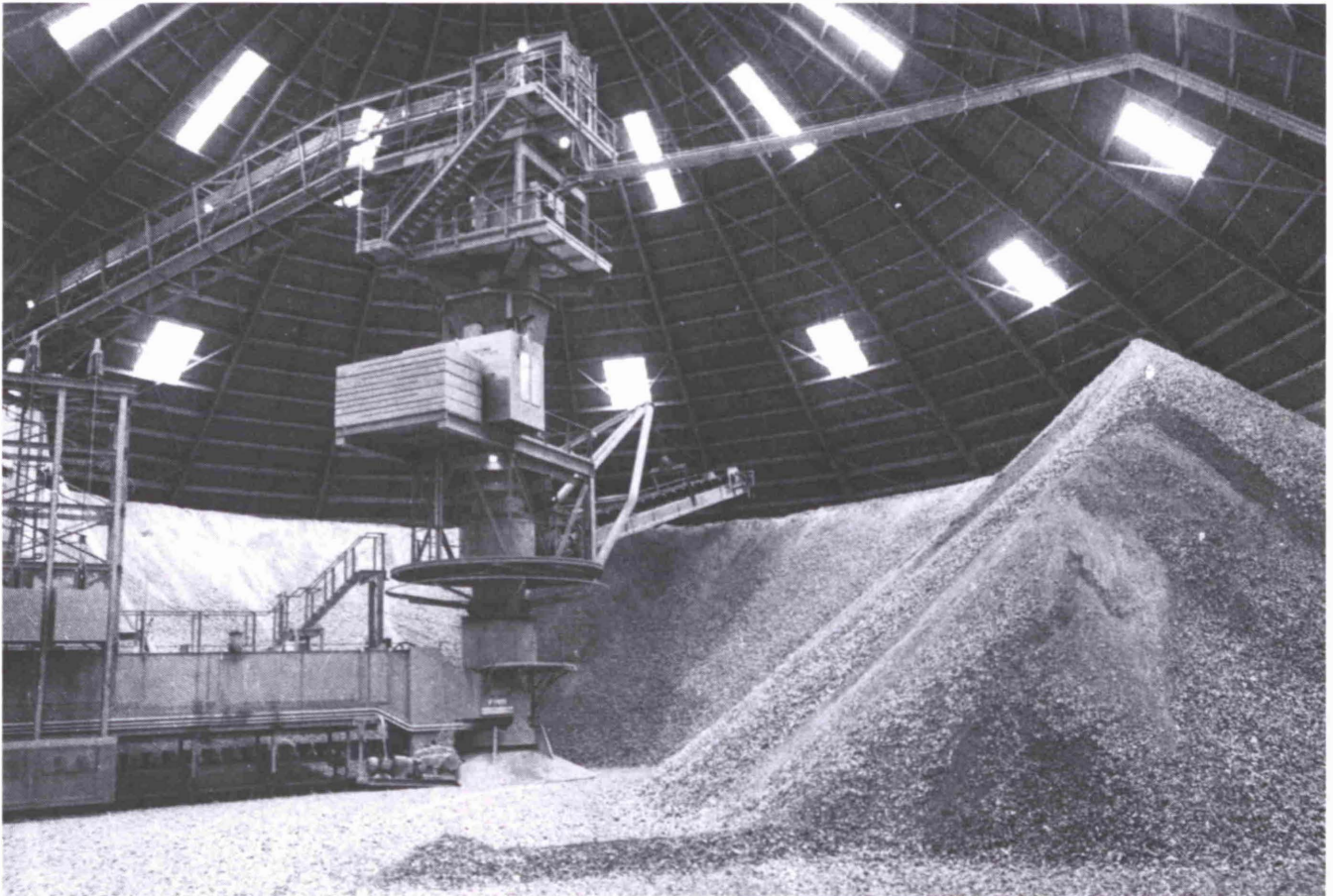
Fig. 3: Circular stockpile with stacker and bridge scraper reclaimer at Redding, California
