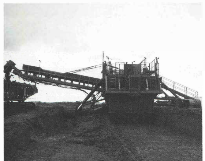
Fig. 3: RAHCO mobile bucket wheel excavator. This unit excavates in both the forward and reverse directions. TMC at left receives and conveys the wet clay
