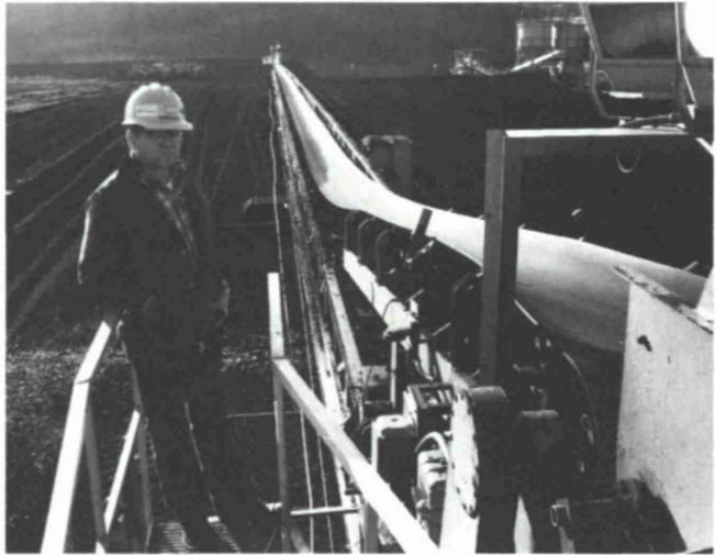
Fig. 5: View from tripper along RAHCO 200 m TMC showing precise support structure alignment and leveling achieved with automatic control systems
