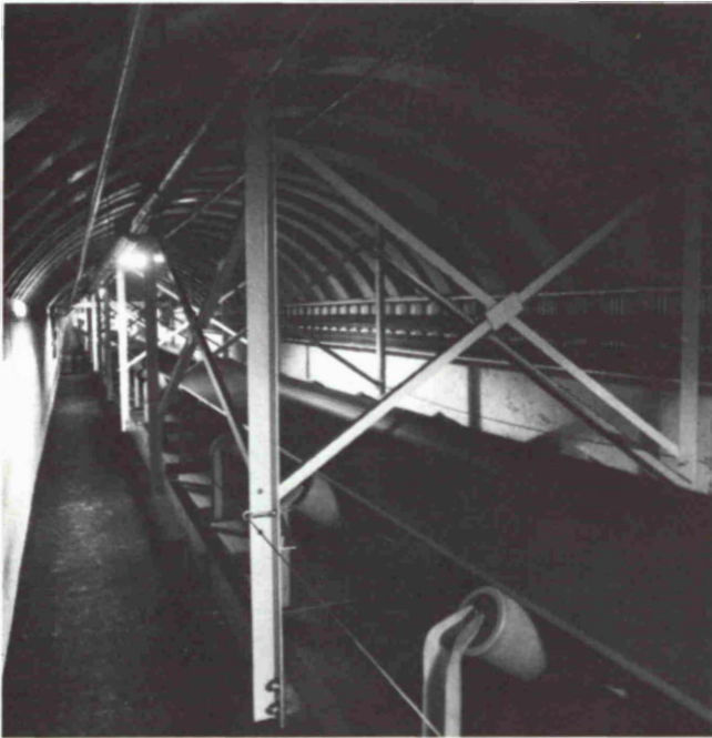
Fig. 3: Section of the 1,200 mm wide conveyor in the tunnel under the river
