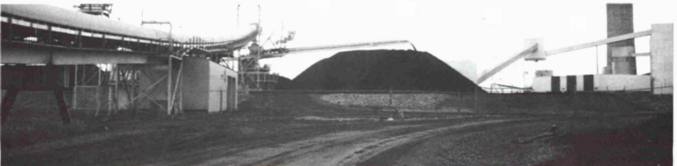
Fig. 5: View of the head end of the overland conveyor and the 40 m boom slewing stacker at the thermal power generating station
