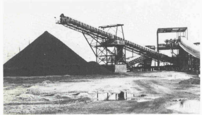
Fig. 11: One of 2 reclaim pits with one trainload live capacity is fed by a fixed stacker at the head end of the yard conveyor
