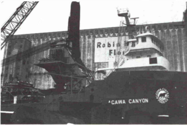
Fig. 6: The FLEXOWELL belt is lowered in an opening in the top part of the elevator casings onto the already erected stub idlers
