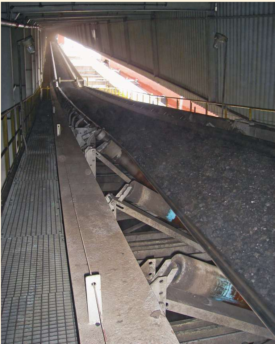
When a chute plugs up, the material spills onto the floor and around the conveyor idlers.
