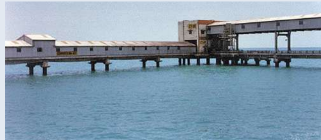
The total distance of between the terminals and the power plant is covered conveyors, each having a length of maximum 1000 metres.
