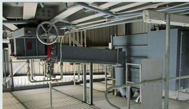
Fig. 3: Silo discharge chute and Dantherm dust control unit.
