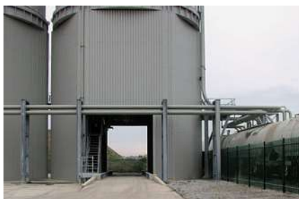
Fig. 1: The rail wagons are connected to the silo inlet pipelines.
