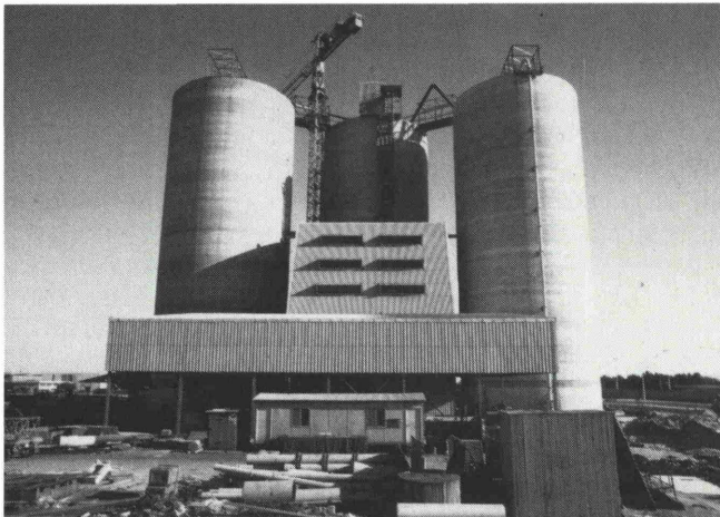
Fig. 5: The three silos of the cement terminal with a storage capacity of 10,000 m 3 each (view from the north)
