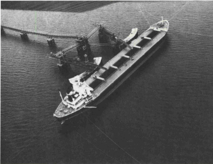
Fig. 4: Dual Radial Loader installation of Soros design at Port Latta for 100,000 DWT ships
