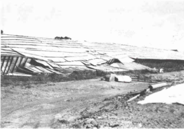
Fig. 10: Collapsed walls of 'A' frame storage
