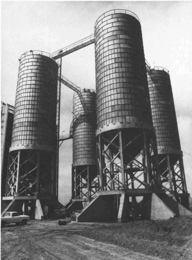
Fig. 3: Silo terminal for 10,000 tons cement capacity in erection. The photo shows the erection scaffoldings and the electrical hoist which runs on the upper edge
