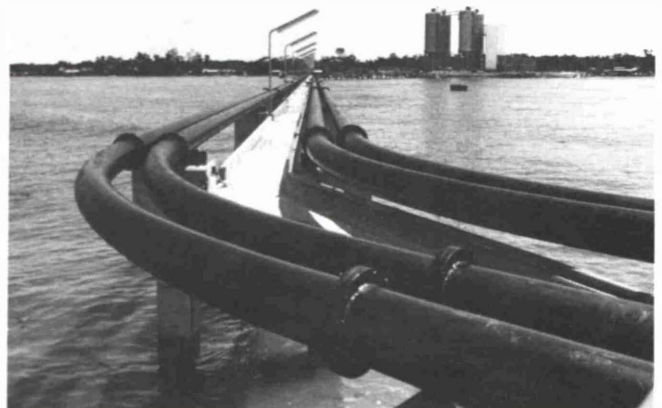
Fig. 2: Feed pipe lines to blow cement into silo station in Venezuela
