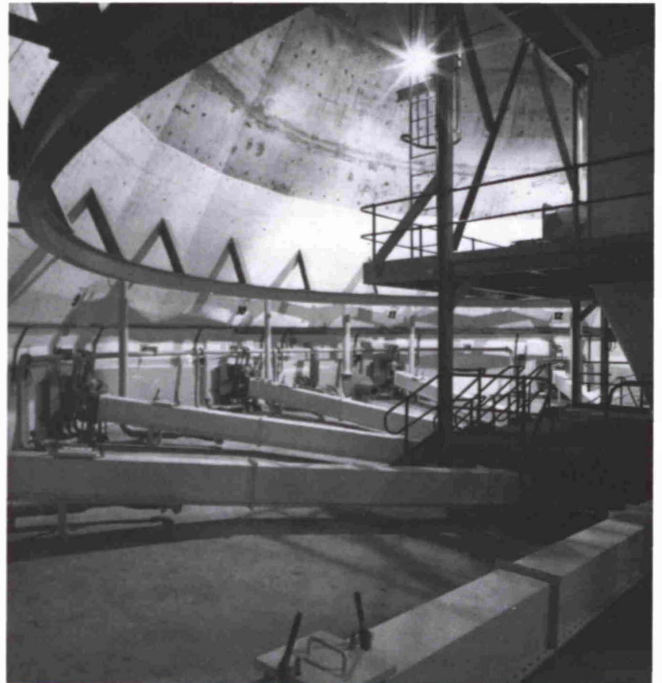
Fig. 8: Two of the 12 silo outlets
