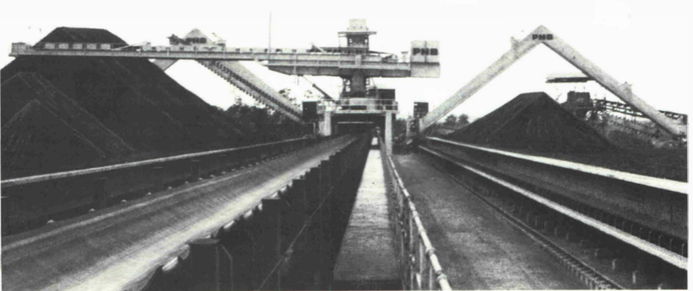
Fig. 6: Thiess Bros. Pty. Ltd. Blackwater Mine coal handling plant including PWH travelling, slewing and luffing stacker and two portal scraper reclaimers
