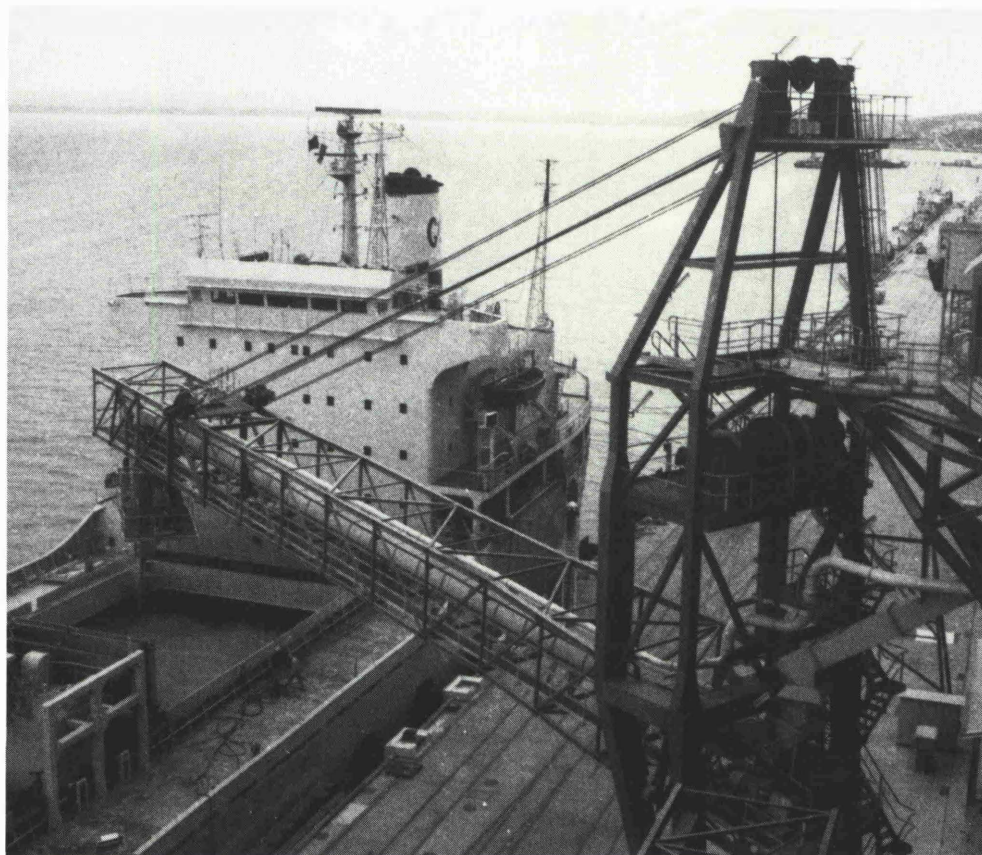
Fig. 5: Fixed position shiploaders at Albany Terminal, Western Australia, each capable of loading ships at 1,000 t/h.
