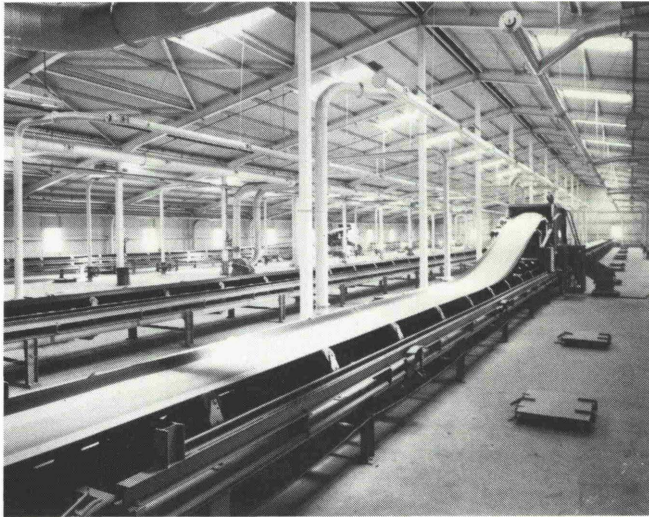
Fig. 4: Oversilo conveyors at Newcastle Terminal, N.S.W. Shows manually operated belt tripper and inlets to storage cells.
