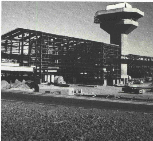
Fig. 7: TS-5 and control tower. Conveyors are elevated, with concrete floors and walls, for washdown. Ground floor has unrestricted access for clean-up.
