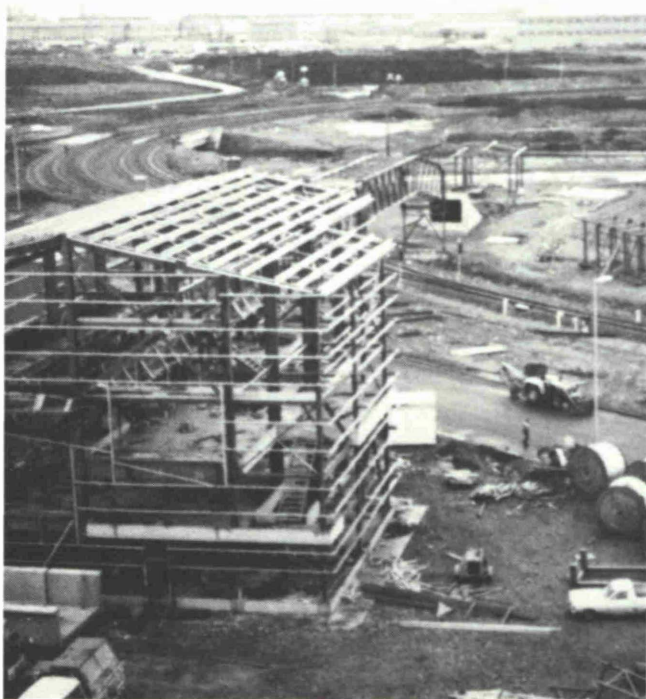
Fig. 3: View of TS-2 with railroad loop and 3-lane truck ramp loading to top of slot storage
