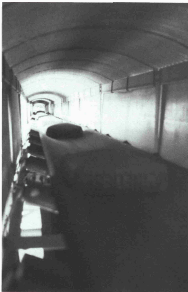
Fig. 9: Belt conveyor system for sacks of cement
