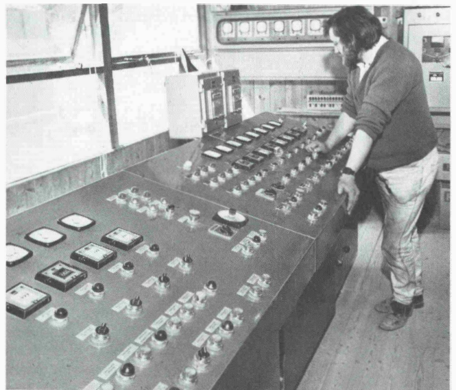
Fig. 4: Rail loading hopper control room at Foster Yeoman, England. Bin-Dex indicators show material levels in the main storage bunkers
