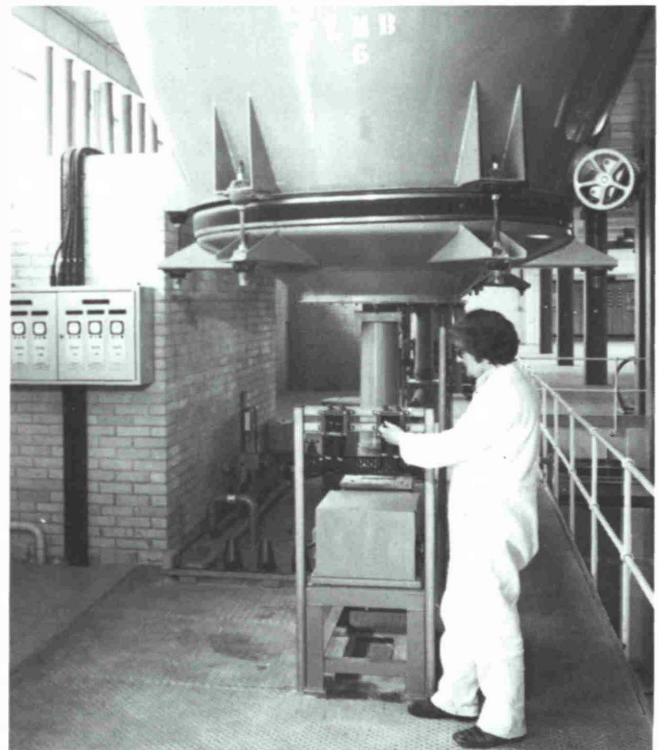
Fig. 1: Bin-Dex repeater indication of chemical levels at the Hanningfield Water Treatment Works, England
