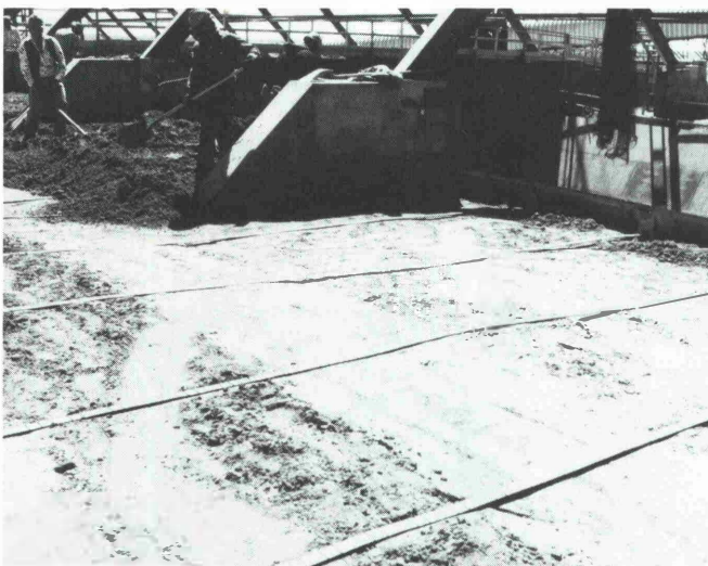
Fig. 11: Spreading backfill around the footings for the roof bents at the Pawnee slot
