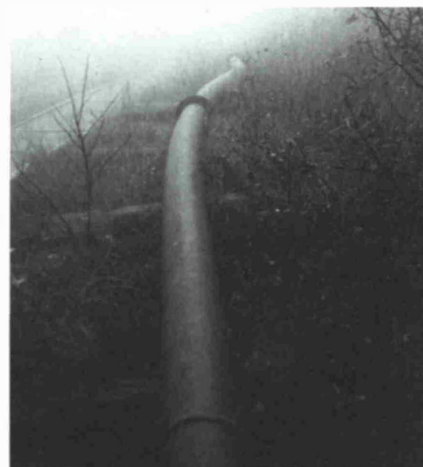
Fig. 9: Transportation of coal pulp in HDPE pipeline
