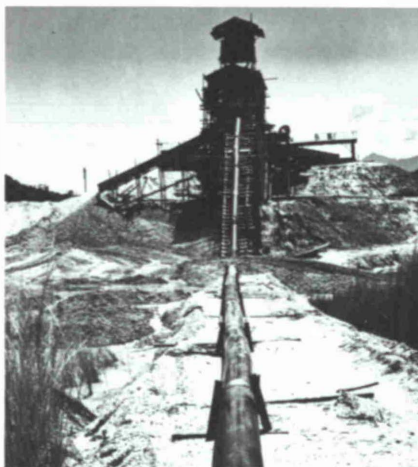
Fig. 8: HDPE pipes made from Hostalen GM 5010 T2 for conveying tin ore water slurries in Malaysia
