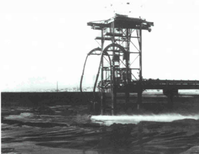
Fig. 3: Mohave Generating Station, near Laughlin, Nevada, employs three basic slurry systems: Pipeline transportation system, storage and slurry reclaim and slurry feed.
