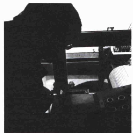
Fig. 7: Operator at dockside control station monitors coal loading operation
