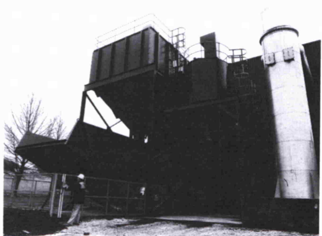
Fig. 2: Auto-Tipper and storage hopper
