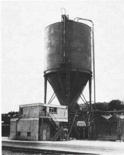
Fig. 1: View of the 1500t storage and transfer complex with the control room in the foreground
