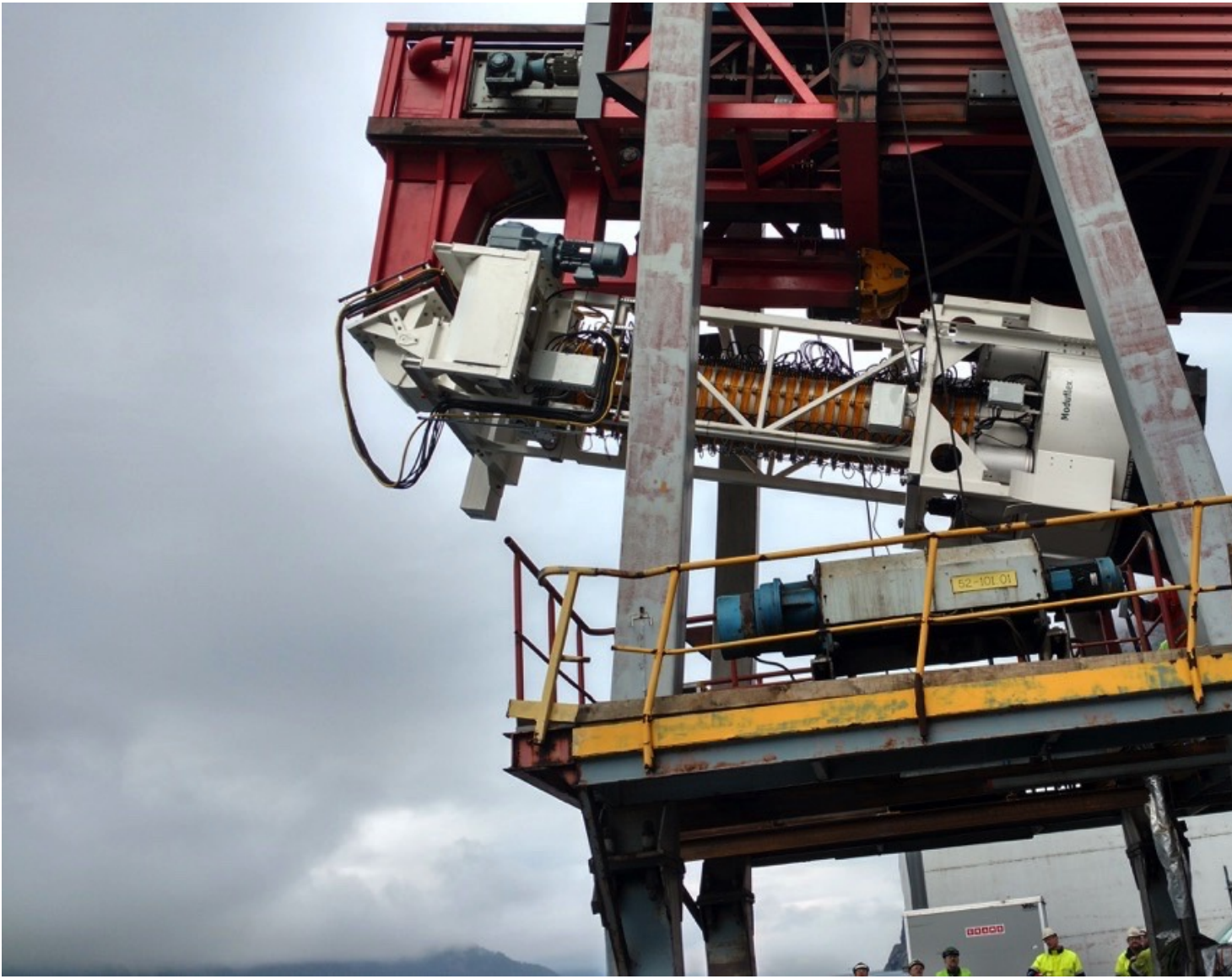
Loading chute with tilting mechanism.
