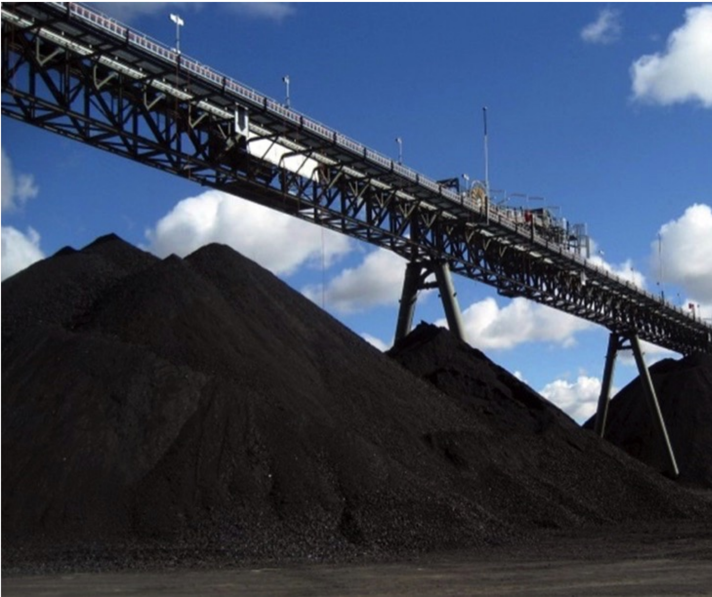
Fig. 1: Coal stockpile with trestle legs supporting the conveyor (Pictures: ©The Authors/TUNRA Bulk Solids)
