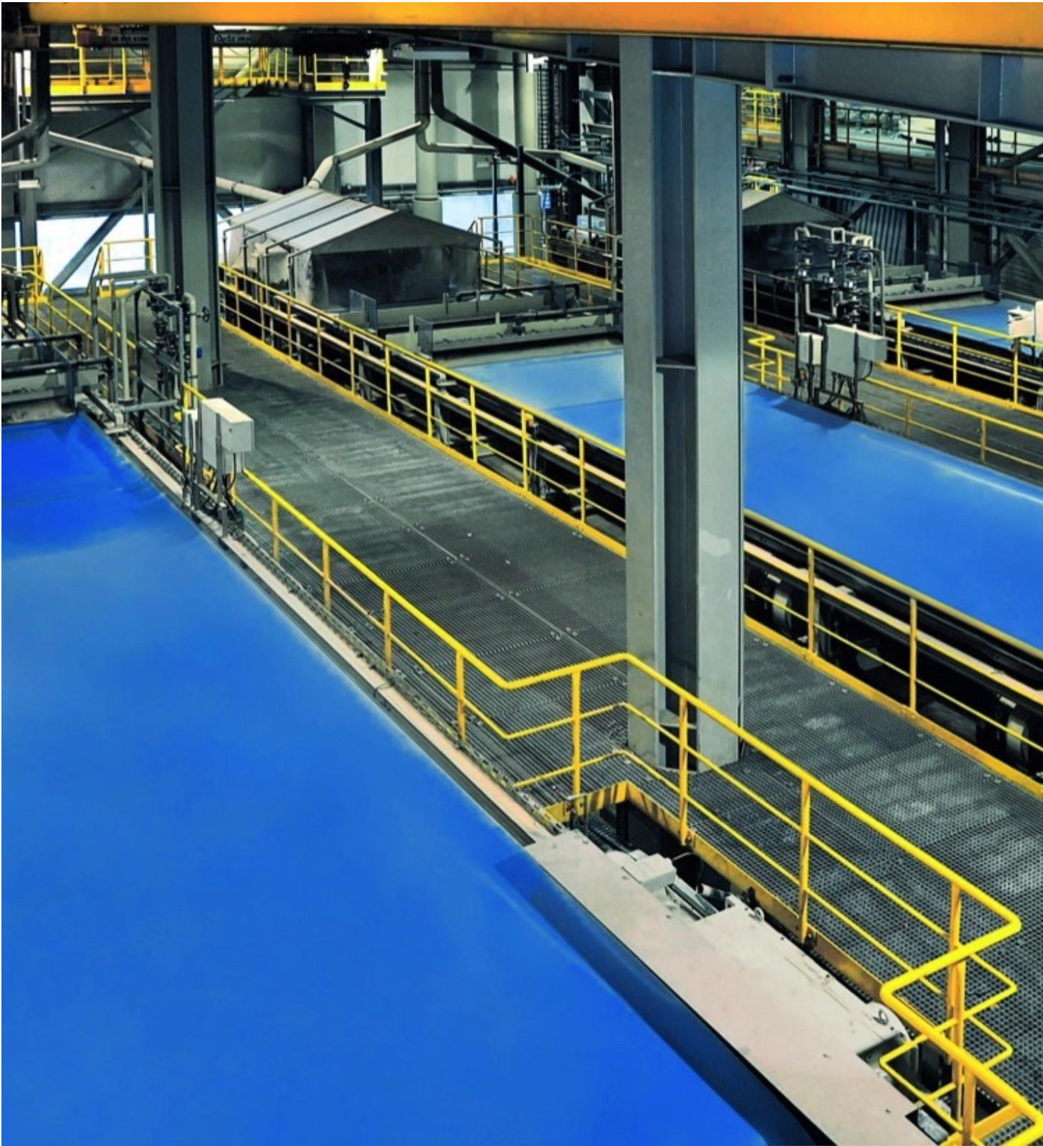
Vacubelt filter belt from GKD for the dewatering of phosphogypsum. (Picture: © ThyssenKrupp Fördertechnik)
