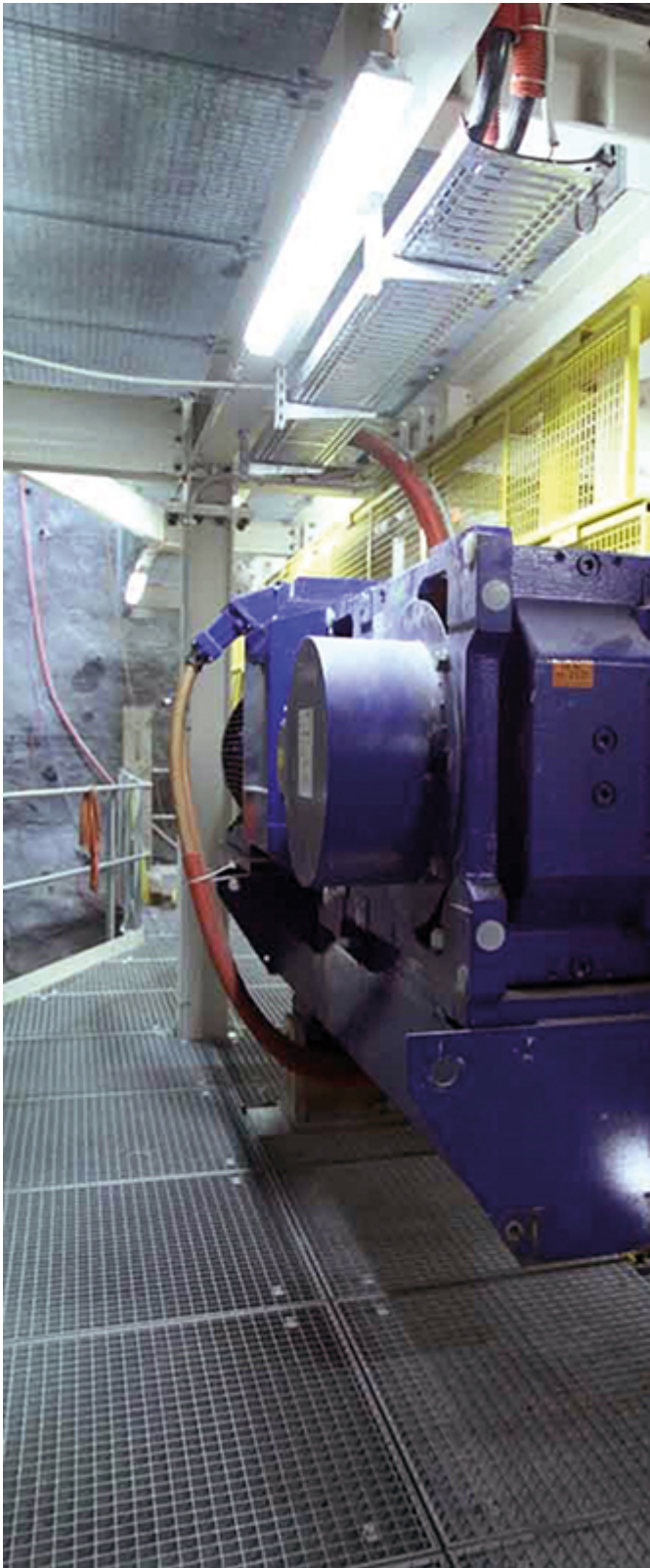
One of the two SK 12407 industrial geared motors that were used to drive the belts; the NORD design allows mounting on all six sides, providing maximum flexibility.
