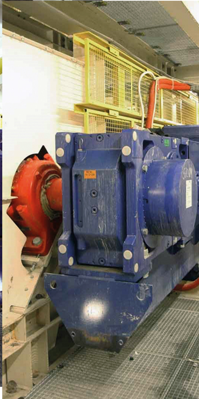
The other of the two SK 12407 industrial geared motors that were used to drive the belts.
