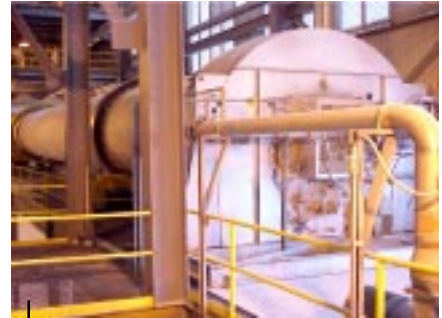
Direct-Fired Rotary Kiln for Calcining Bauxite
